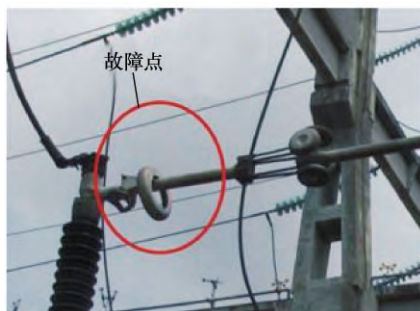
(a) 故障点情况
