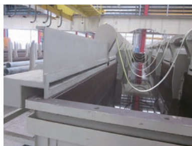
(a) 酸洗槽四周设置抽风槽
