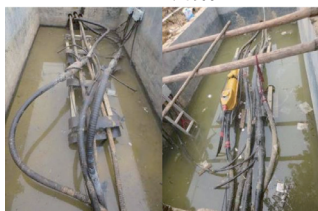
(a) 1#电缆井 (b) 3#电缆井
