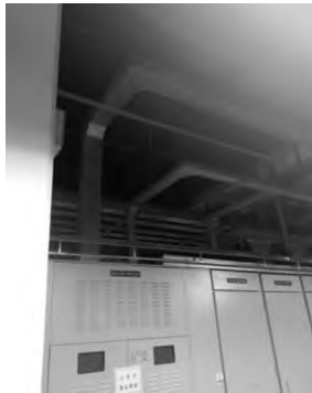
图4 变电柜上方桥架现状 Fig. 4 Current situation of the bridge above the transformer cabinet
