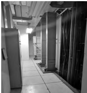
图3 现场电井 Fig. 3 Field electric well
