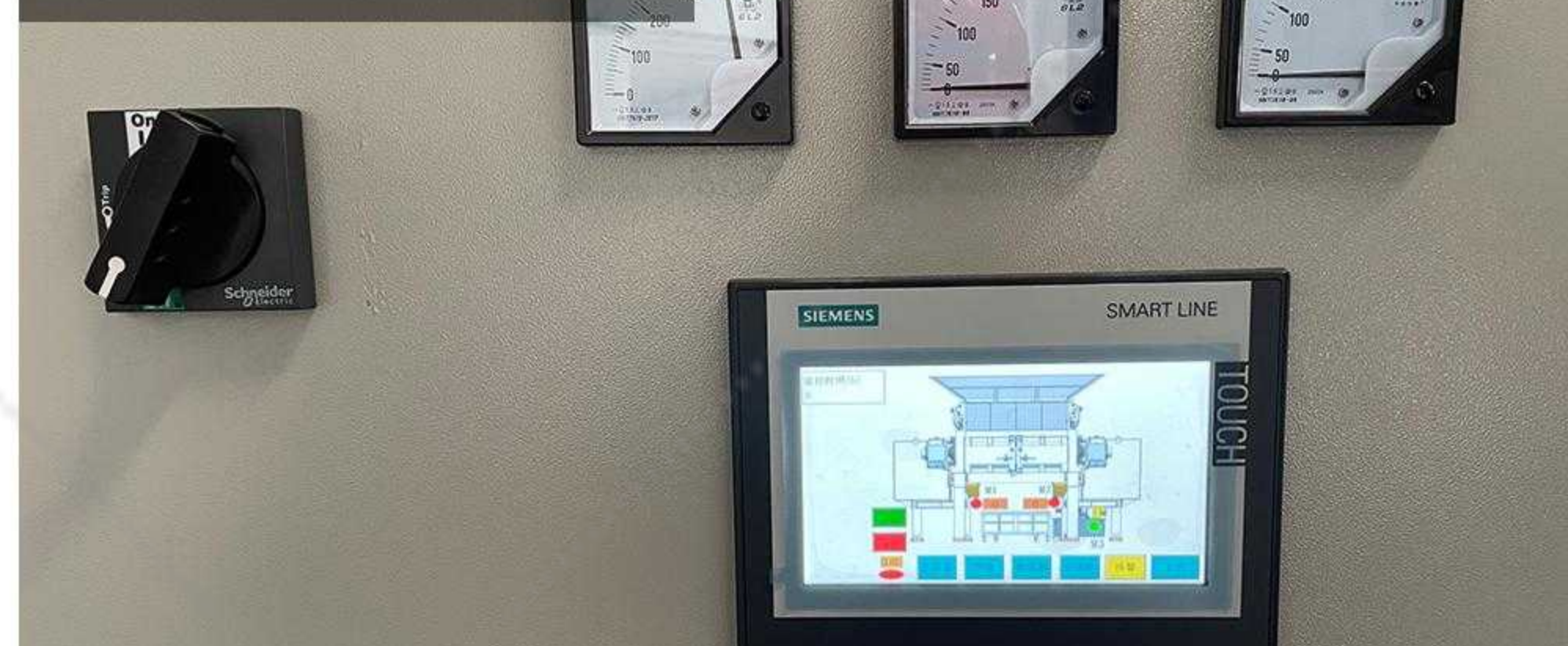
电控 Electrical Control
